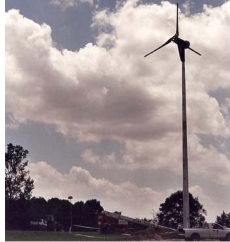
SunWind Power Systems installs 15 kW wind turbine for Hoosier Energy.
