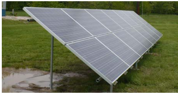
1b) Ground mount 3 kW PV system in Merom, IN
