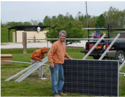
Figure 1a) Jeremy Coxon, mechanical engineer, is the project manager for the solar install at Turtle Creek.
