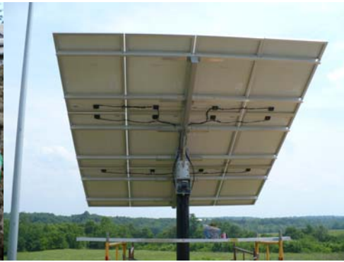
Pole Mount Solar PV Panels
